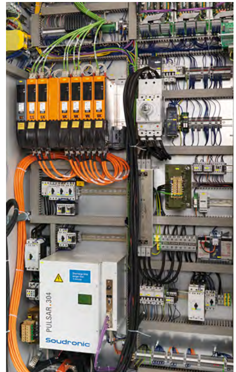
UNICONTROL control system and PULSAR static frequency converter
